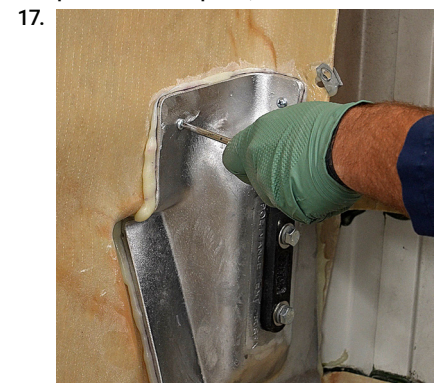
Screw the casting to the hood. On preventative repairs, the OEM bolts should be installed before tightening the screws and elevator bolt.
