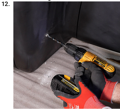
Counter-bore the 1/4" hole, 1/4" deep with a 3/8" drill bit to provide clearance for the bolt's shoulder. Tap the elevator bolt with rubber washer into the hole.
