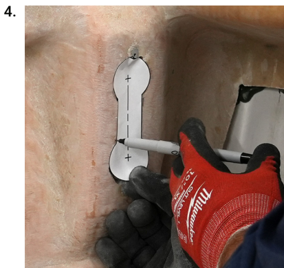
4. On preventative installations, remove the bolts then heat the fork until the adhesive is soft, pry off. Trace the paper template and grind the fiberglass down to the metal plate.
